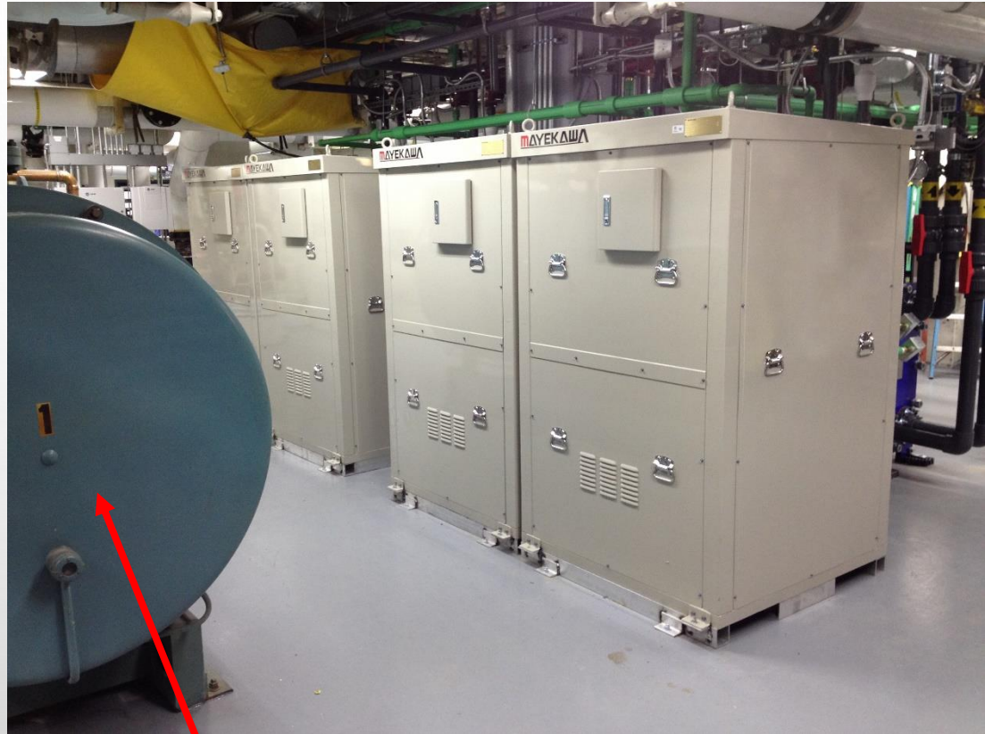
Existing Oil Boiler
